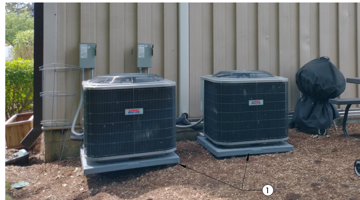
EXISTING BUILDING – COMPRESSORS
